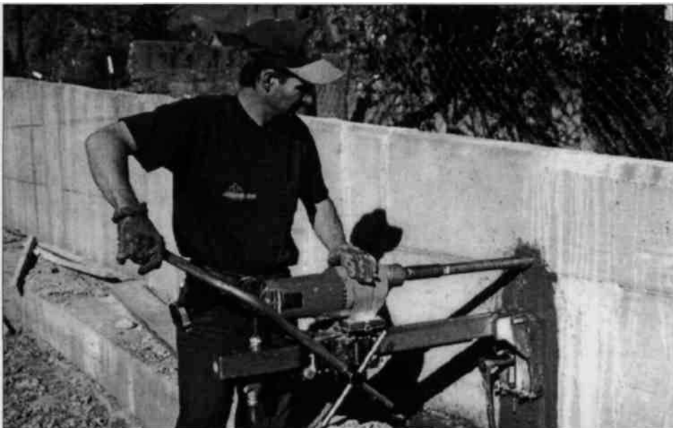
The drill is shown here cutting a "weep" hole through a concrete wall. The hole is necessary to relieve water pressure against the wall which could eventually push it over.
